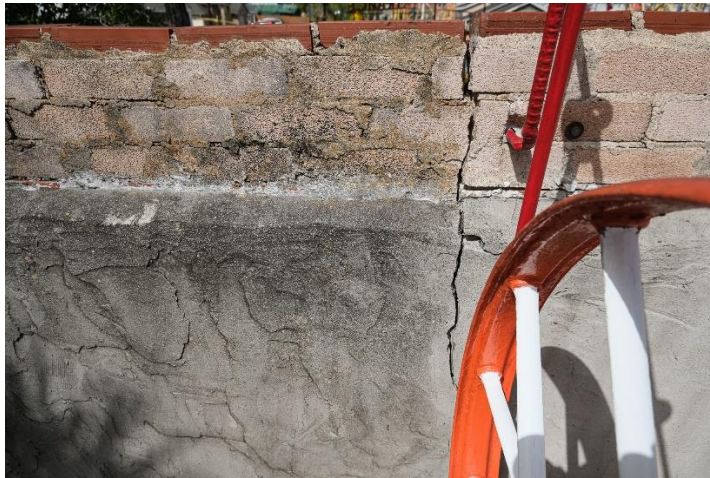
Figure 36. Crack on second floor observation deck behind side stage.
