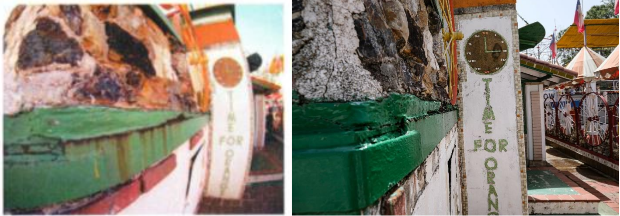
Figure 31. Perimeter framing angle is sandwiched between layers of masonry, promoting corrosion (left:2012, right: 2021).
