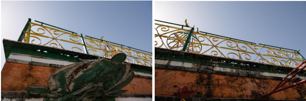
Figure 39. Observation deck showing corrosion in steel at perimeter.
