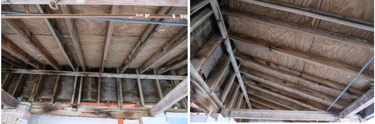
Figure 38. Wood decay at Side Show stage ceiling.
