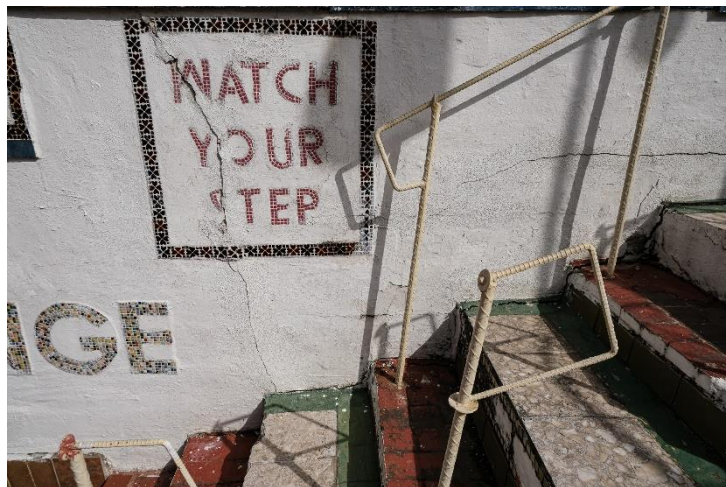
Figure 37. Crack along east wall of Amphitheater seating.
