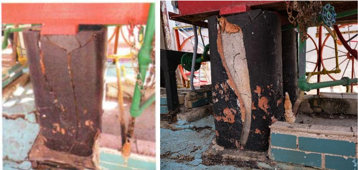
Figure 32. Corrosion expansion cracking a characteristic post-base made of hollow tile and filled with mortar. (left:2012, right: 2021)
