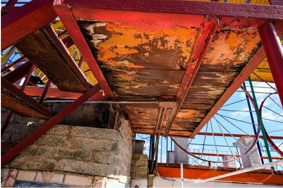
Figure 33. Wood decay and corrosion at the underside of stairs.
