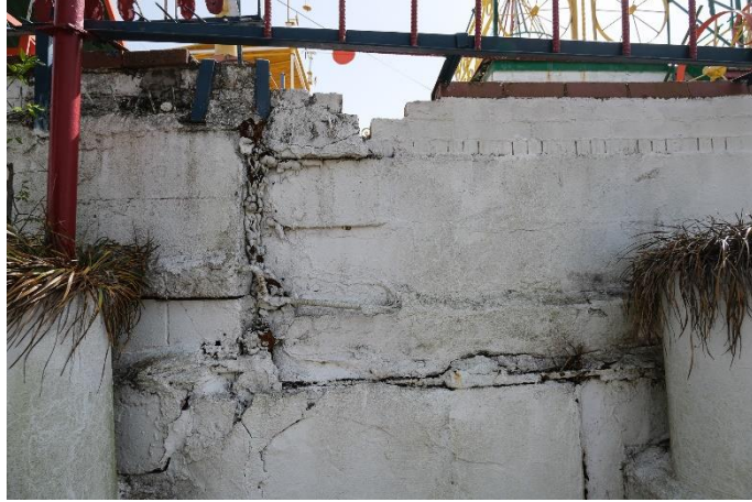
Figure 35. Crack along north exterior wall.
